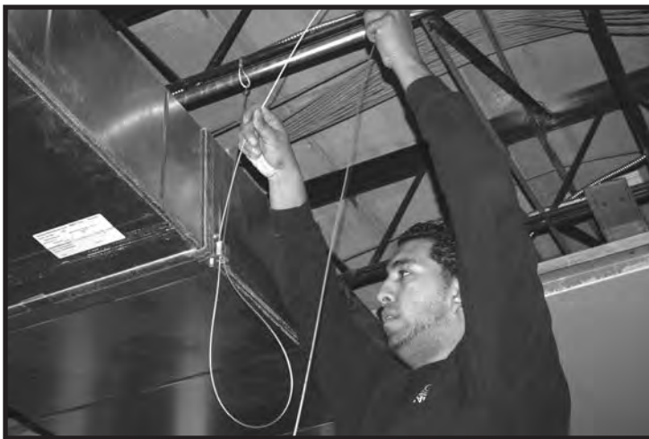
Installation of the KV Bracket at the Elmont Library in Nassau County, NY
