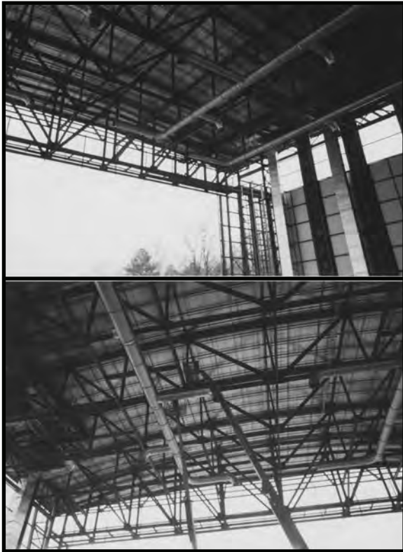
Spiral Ductwork hung by Dyna-Tites (above and at right)
