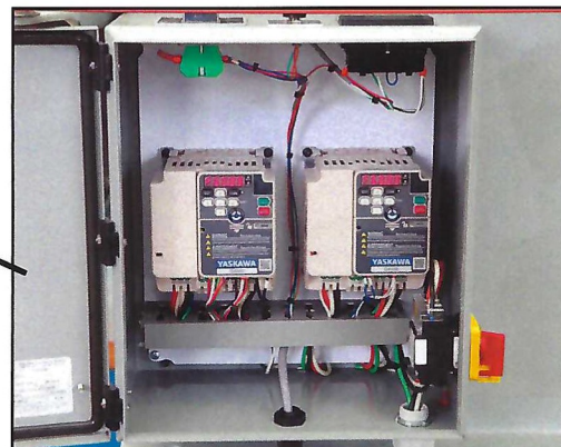
Electrical enclosure with variable frequency drive. 3 phase 230/460 volts NFPA-79 specifications 24 VDC control circuit Overload protected
